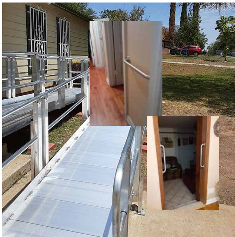
A Ramp and Grab Bars Were Installed For Ms. Norma Martinez's Home
