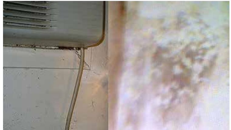
Mold condition at Mr. Paul Fox' apartment
