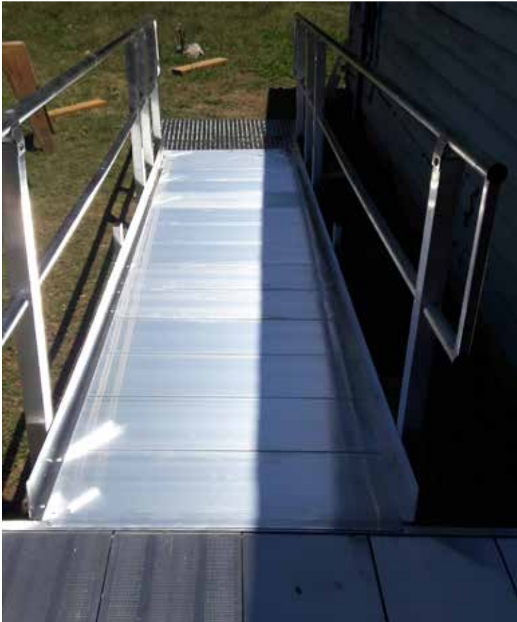
An access ramp was installed at Samuel Cuellar's home, it is a life saver
